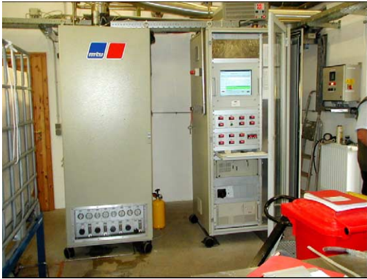
Fig. 1. MCFC testbed (left: MCFC unit; right: controlling unit).
